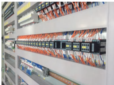
■ PLC柜 PLC Cabinet
